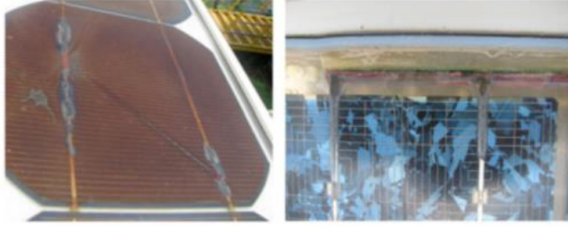
Figure 2.4: Corrosion in interconnections and metallic contacts of two different modules [5]
